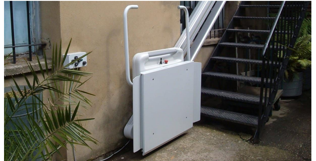
Platform stair lift
