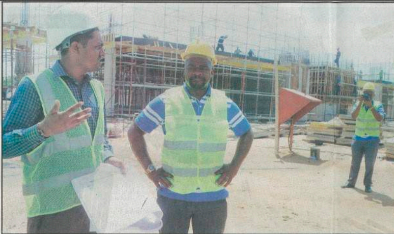
National Housing Corporation director general Nehemia Kyondo Mhechu (2nd-L) is updated by Kishor Hirani, an engineer with Estim Construction Company, when he toured the corporation's Kawe Beach 711 development project in Dar es Salaam yesterday. (Photo: Mpokei Bukuku)
