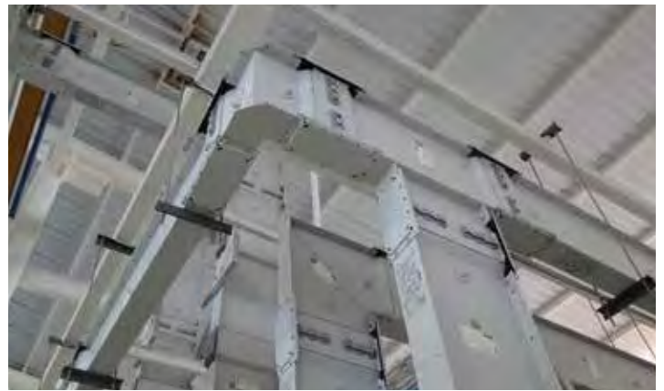
Example of Zucchini busbar system
