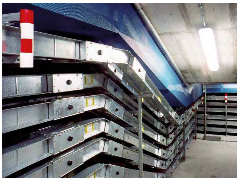
Example of high power distribution
