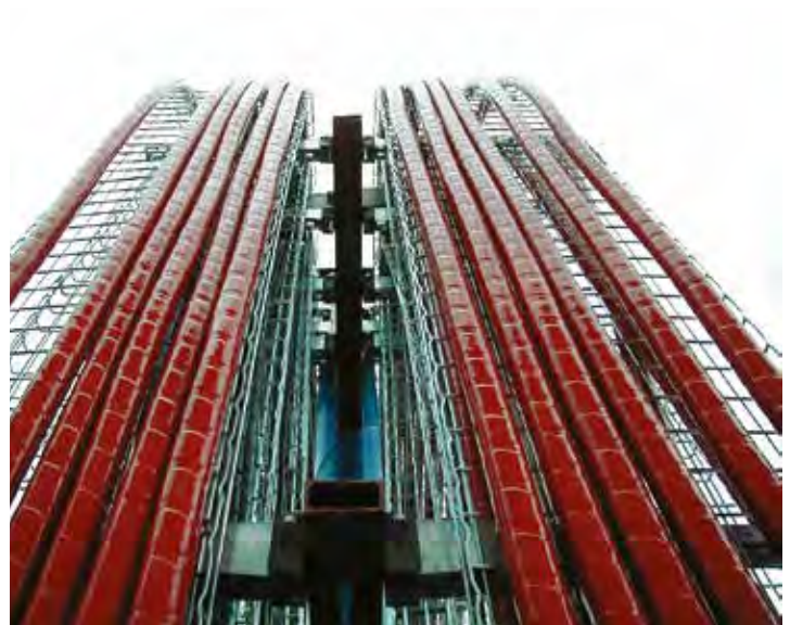
Example of more space busy by cable tray distribution
